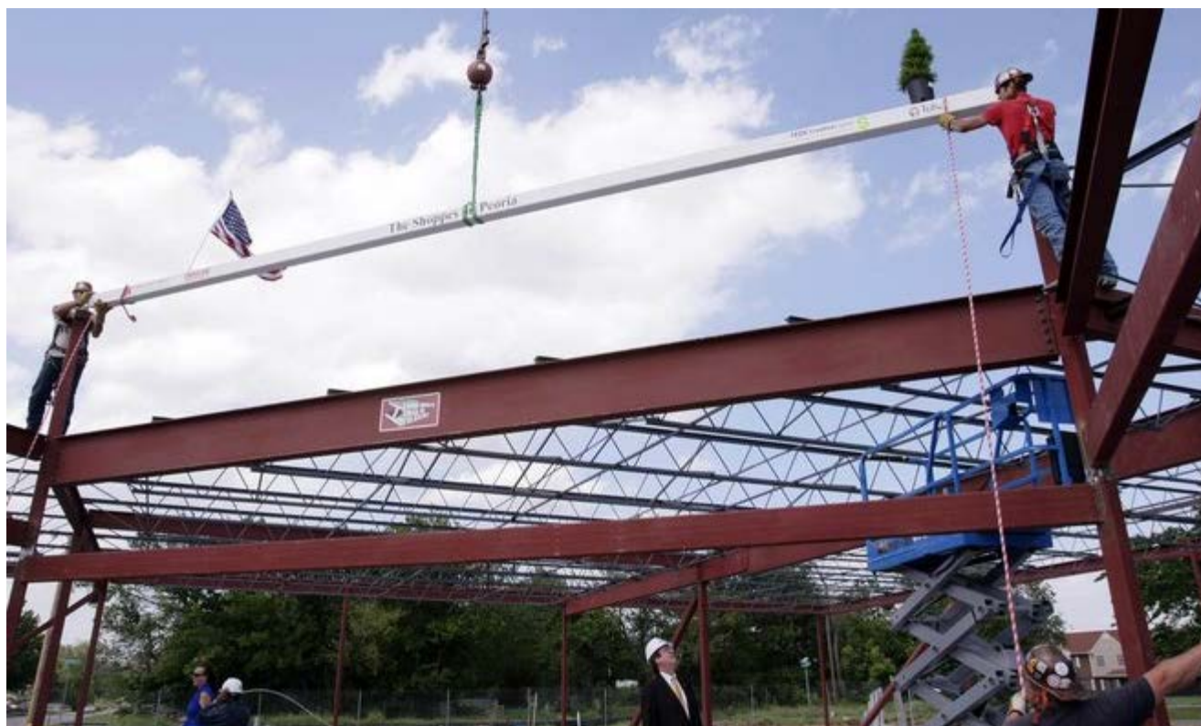
Mayor Dewey Bartlett stands underneath the final beam as workers put it in place Friday at the Shoppes on Peoria project's "topping off" ceremonies. MICHAEL WYKE/Tulsa World
